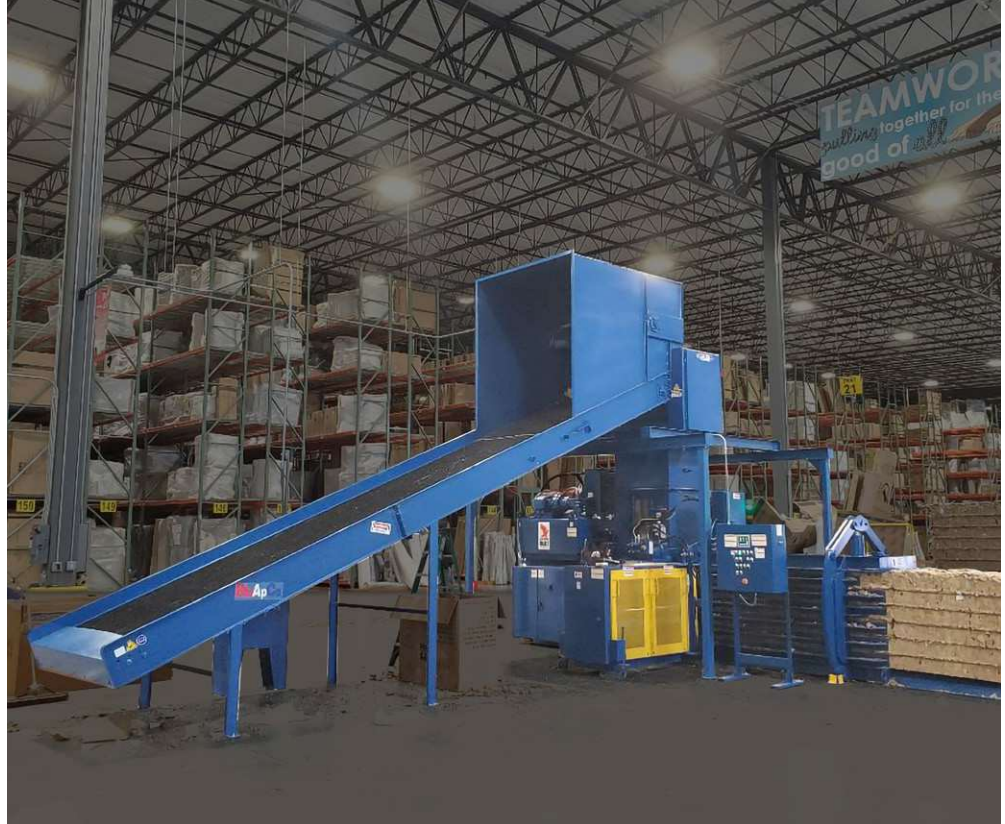
A BloApCo piggyback shredder with a box crusher mounted over a horizontal auto-tie baler.
